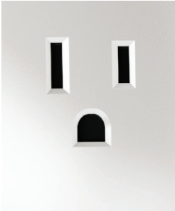
five AC outlets
